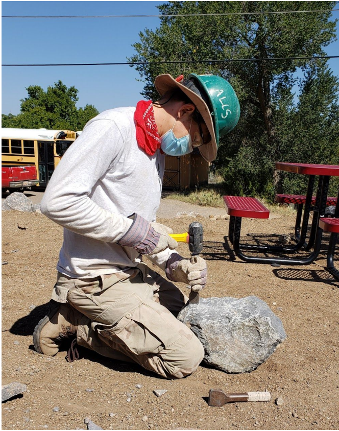
Trail crew is making progress in the Student drop off area. Eleventh grader Colin shapes a rock.
